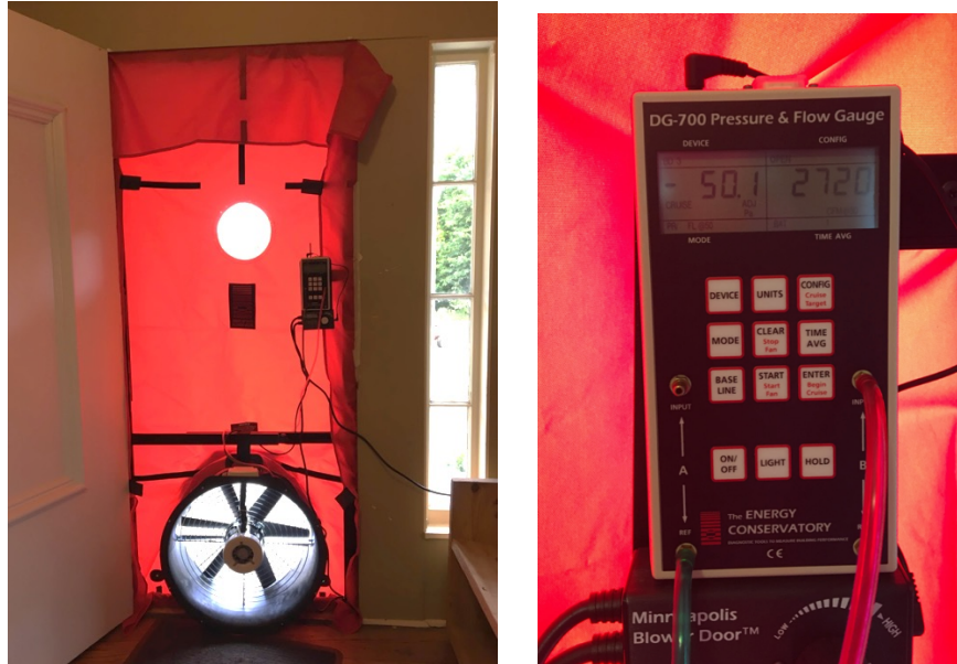
Figure 6: Blower door installed for whole building (left); example screen showing 50Pa building pressure (right)
