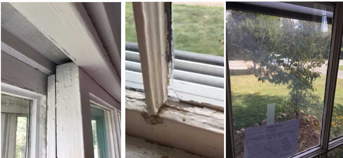
Figure 24: Solarium window gap (left); pane glass crack and deteriorating caulking (middle); pane crack (left)
